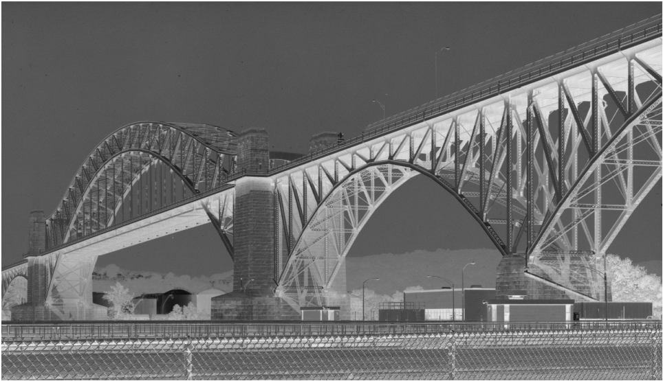
Figure 19.2: The McKees Rocks Bridge in McKees Rocks, Allegheny County, Pennsylvania, built in 1931, is listed on the US National Register of Historic Places. Photo courtesy of the Library of Congress, Prints & Photographs Division, HAER, Reproduction number HAER PA, 2-MCKRO,2-1. Photographer: Joseph Elliott, 1997.
